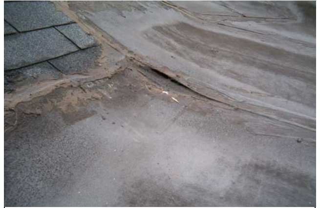
rear roof - Seam open...
