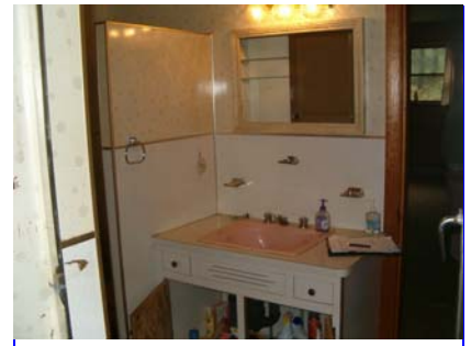
Check flooring near toilet
