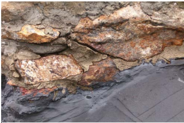
cracked mortar in chimney...
