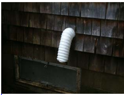
Needs vent cover
