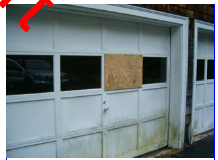
broken garage window
