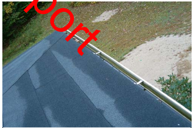
Leaking gutter in center span....
