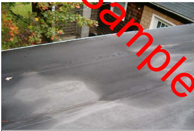
Spongy area over rear flat roof...
