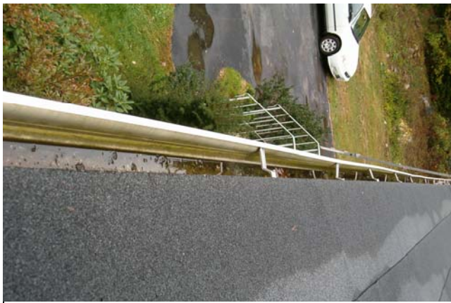
gutter not pitched correctly....
