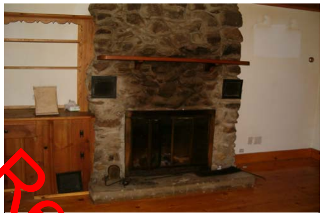
Smoke stained chimney..
