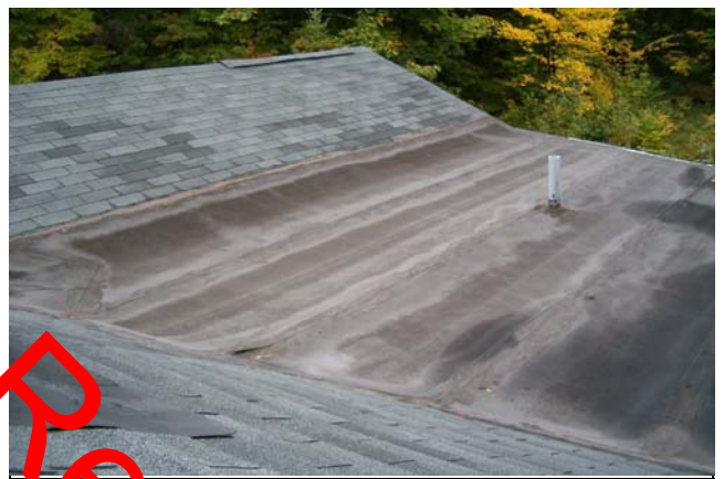
Improper roof installation....
