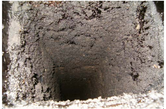
Chimney in serious need of a cleaning..
