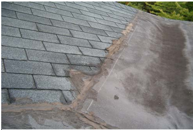
Improper valley installation...
