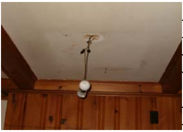
Hanging light fixtures
