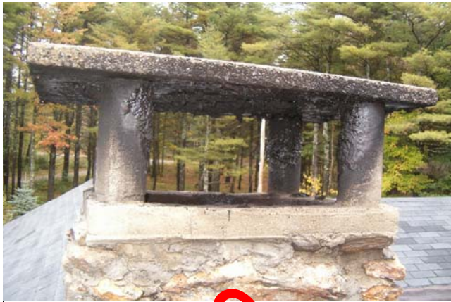
Chimney not high enough..
