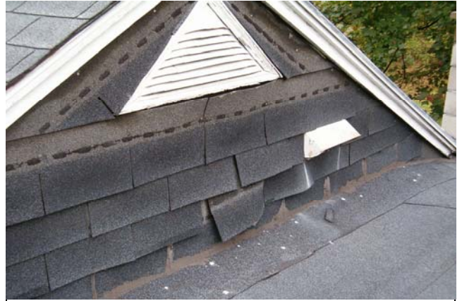
Shingle falling off and missing....
